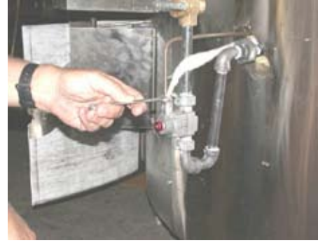
2. Using a 3/8" wrench, remove the brass thermocouple fitting from the safety control.
